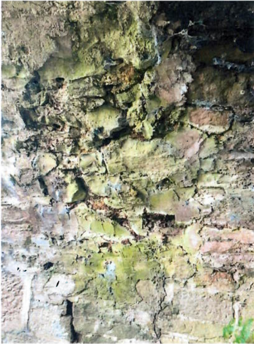
Figure 2. Cracks, holes and deteriorating stone and mortar on the underside of one of the arches.
