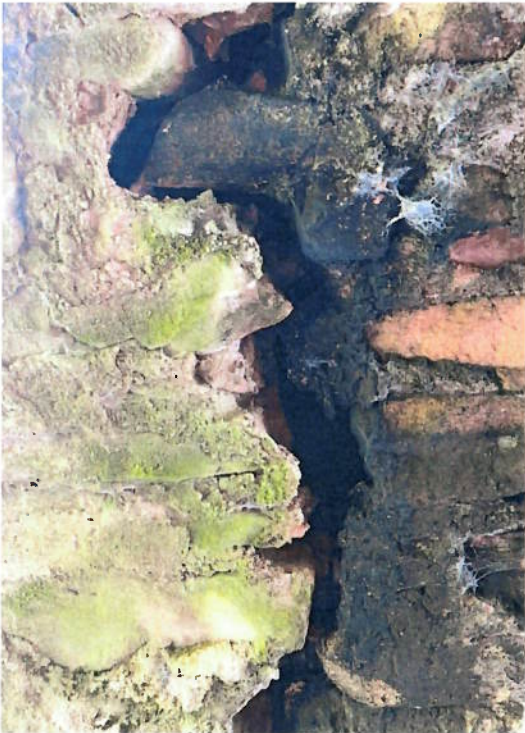
Figure 3. A large crack present on the underside of one of the arches.
