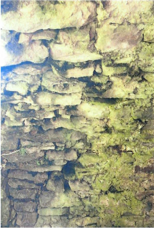
Figure 4. Cracks, holes and dislodged mortar on the underside of one of the arches.
